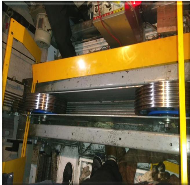
Example of installing a "division independent rope pulley" on top of an L-type lift car
